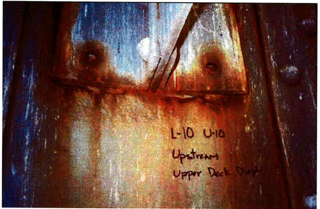
Photo 10: Looking inside L10-U10, upstream truss. Note pack rust has broken two rivets.
