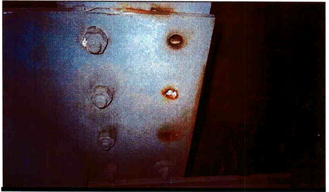
Photo 11: Looking up at gusset plate connecting bottom flange of upper deck floorbeam 9' to the downstream truss. Note \frac{3}{4} inch pack rust has developed in location where 3 bolts are missing.
