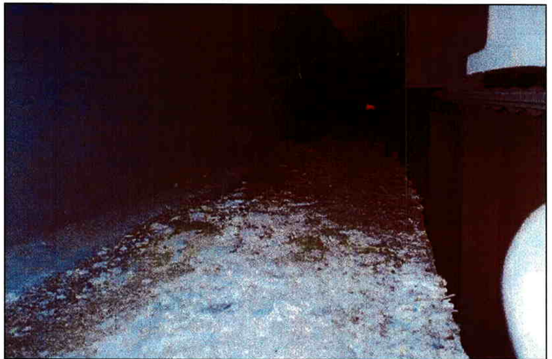
Photo 8: Looking east at drainage trough at Pier IV. Note trough is completely filled and cannot drain into drainpipes.
