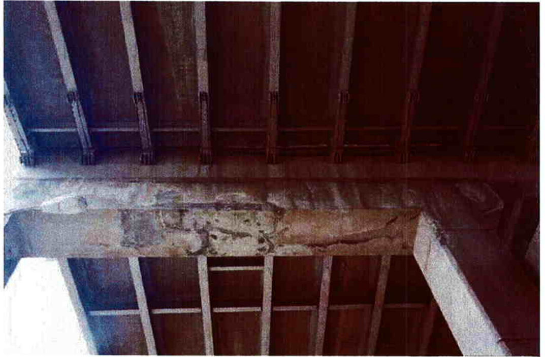
Photo 5: Looking up at Pier 7 in south approach. Note fallen compression seal.
