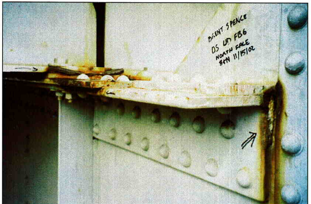
Photo 6: Looking east at downstream north face of upper deck floorbeam 6. Note pack rust under stringer bearings, between top flange cover plate and angles, and between top flange angle and web.
