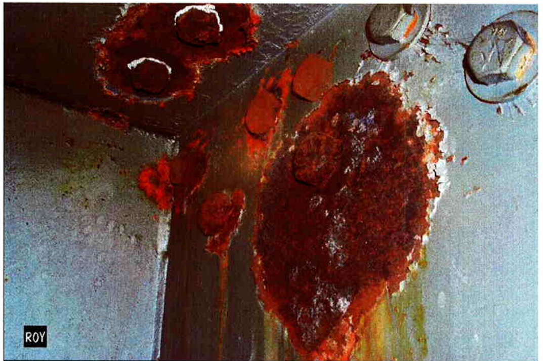
Photo 6: Looking up at misdrilled holes in top flange plate, pier cap at Pier IV. Note corrosion inside cap due to roadway drainage leaking through holes.
