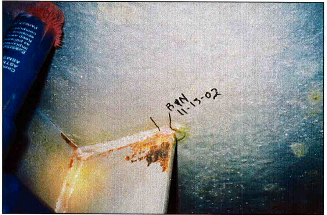
Photo 5: Looking east at west face of stiffener between bearing diaphragm and diaphragm 1 in UD3 pier cap. Note 5/8" crack in top weld.
