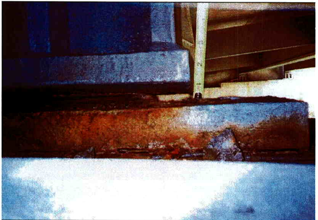
Photo 2: Looking north at bearing for girder 3 at pier H2. Note pack rust under rocker has lifted bearing by \frac{1}{2} inch from masonry plate.
