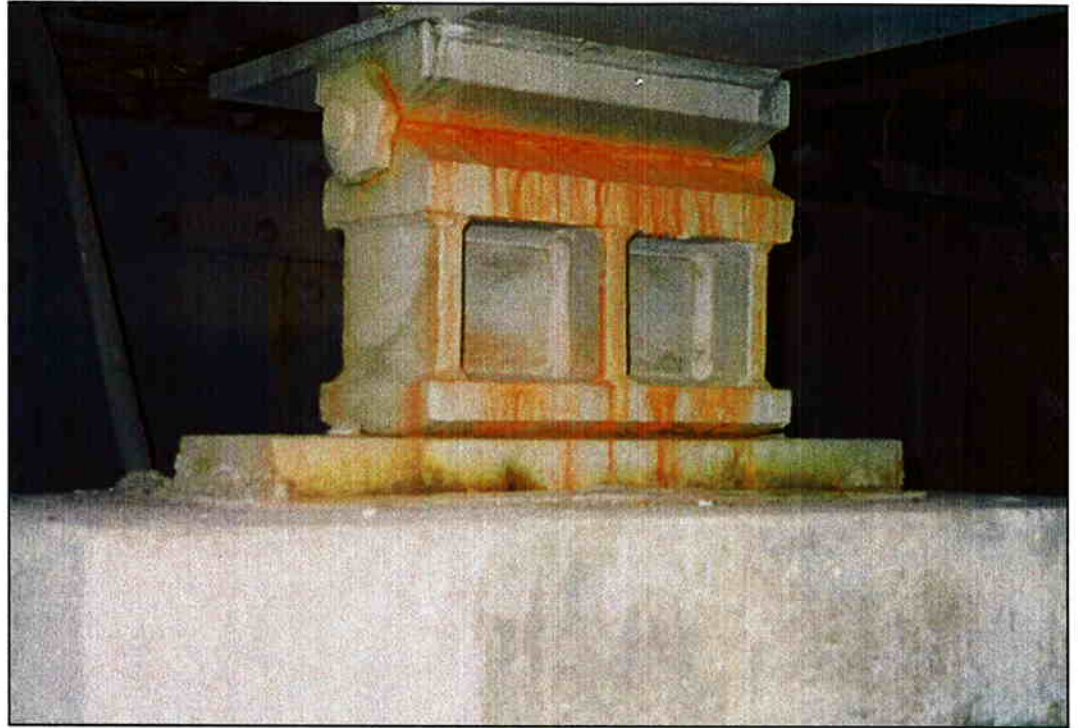
Photo 1: Looking north at bearing for girder 9 on Pier IV, lower deck. Note fretting corrosion on pin indicative of relative movement between girder and bearing.
