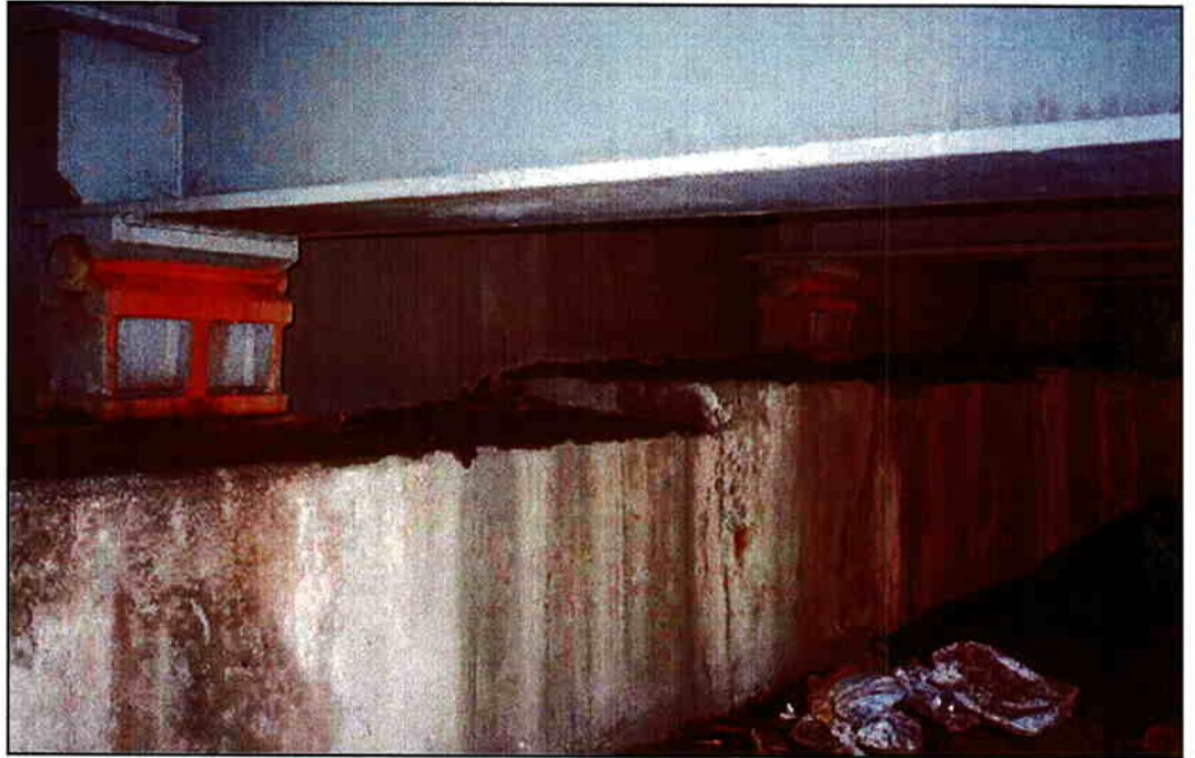
Photo 1: Looking south at bearings for stringers 5 and 6, south lower deck abutment. Note heavy staining from fretting corrosion indicative of lifted bearings.
