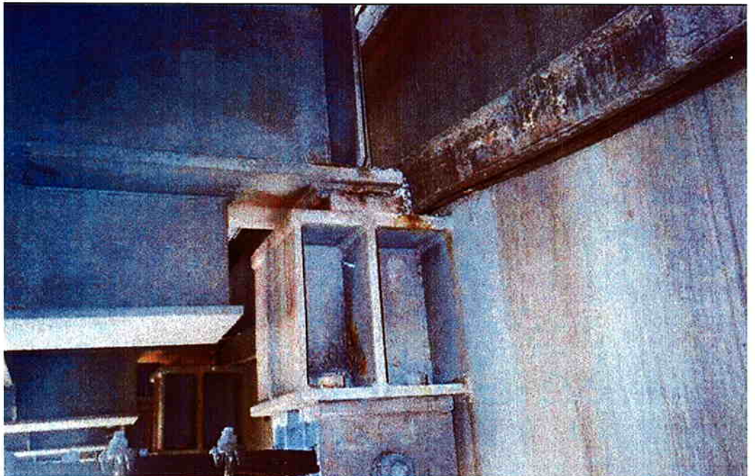
Photo 4: Looking west at stringer 6, south side of Pier Cap 7. Note fallen compression seal and debris behind sliding seat stringer bearing obstructing stringer movement.
