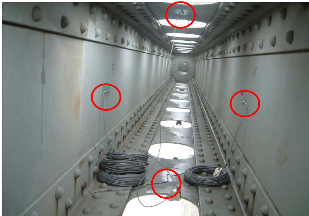
Figure 7. Weldable Strain Gages in Diagonal Truss Member
