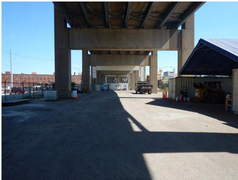
Photograph 10. View of the underside of the Brent Spence Bridge showing no signs of bat usage, looking north.
