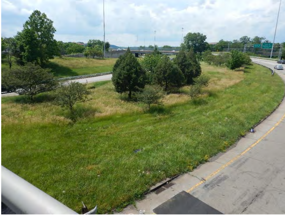
Photograph 35. View of I-75 right-of-way with mowed grass and pine trees, looking northwest.
