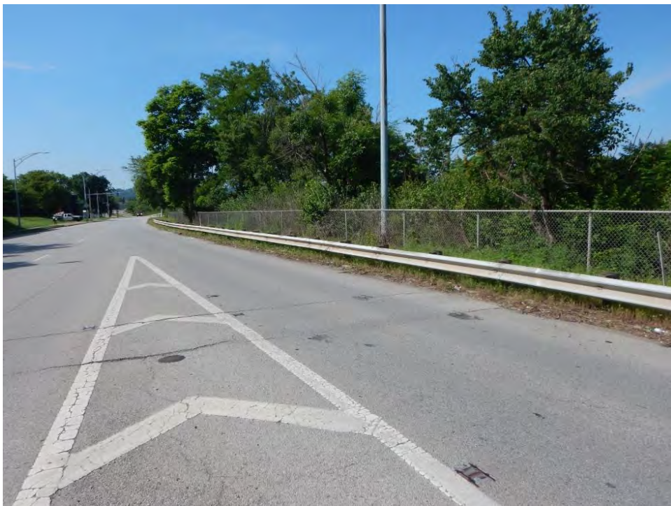
Photograph 88. View along Western Avenue and I-75 right-of-way with SWH (right side), looking north.
