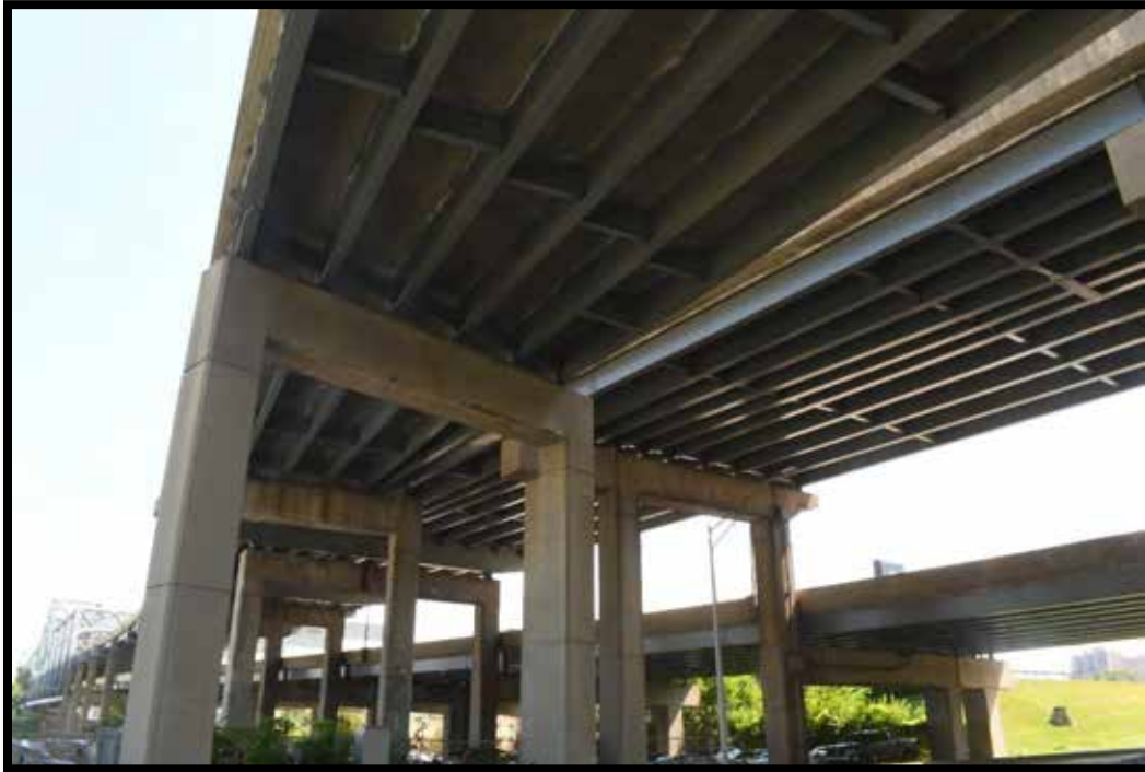
Plate 528. Bridge No. 059B00040N. Underneath decking, girders, and piers of Third, Fourth, and Fifth Street overpass approach of I-75/71 to Brent Spence Bridge (Bridge No. 059B00046N), looking northeast.
