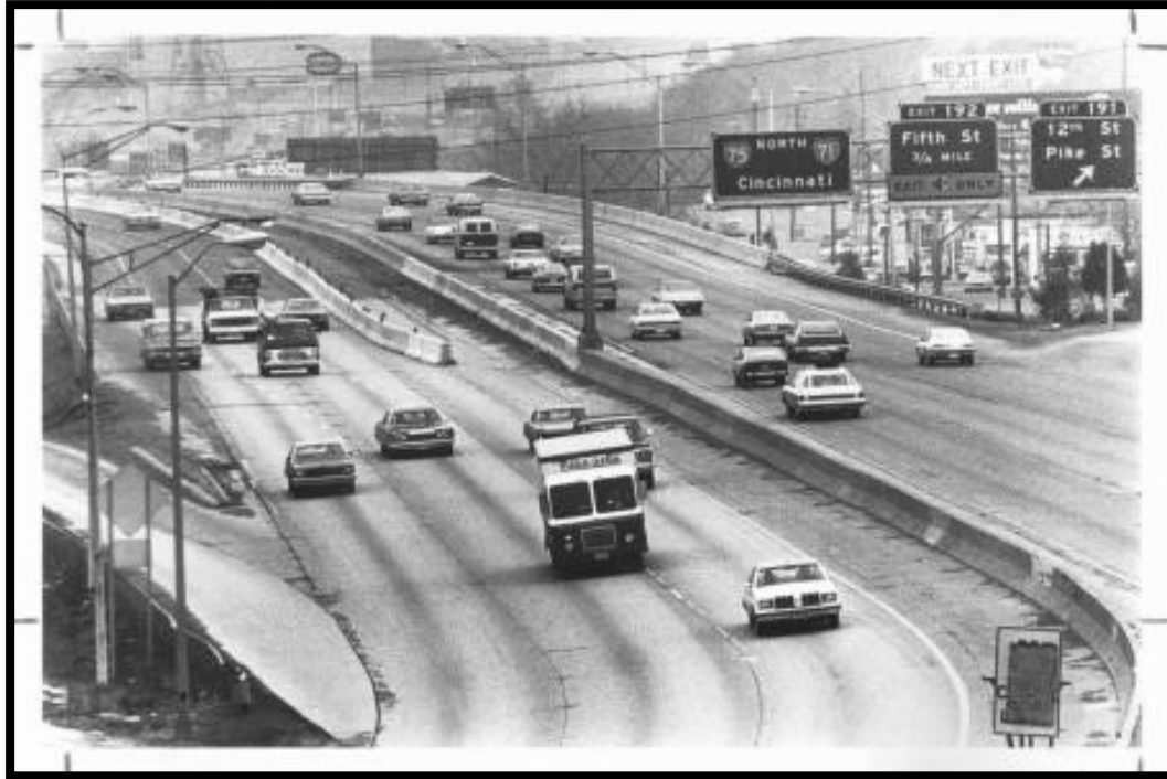
Figure 90. Bridge No. 059B00044R. Photograph depicting this bridge being widened, April 3, 1981, looking north. 470
