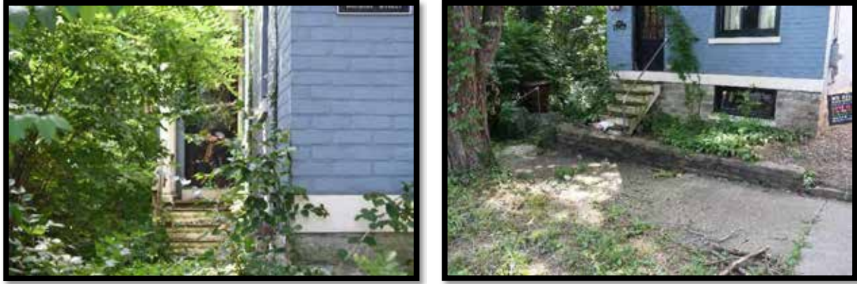
Plate 158. Left: Recessed northeast side entry, looking southeast. Right: Mortared stone wall, looking southeast.
