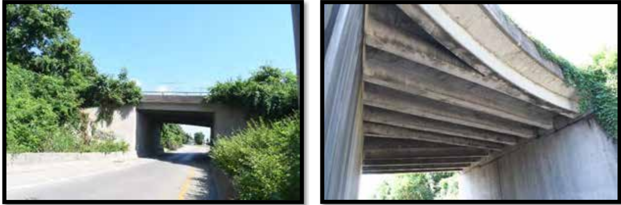
Plate 531. Bridge No. 059B00039N. Left: looking north. Right: Underneath view of concrete piers, girders, and decking, looking SW.
