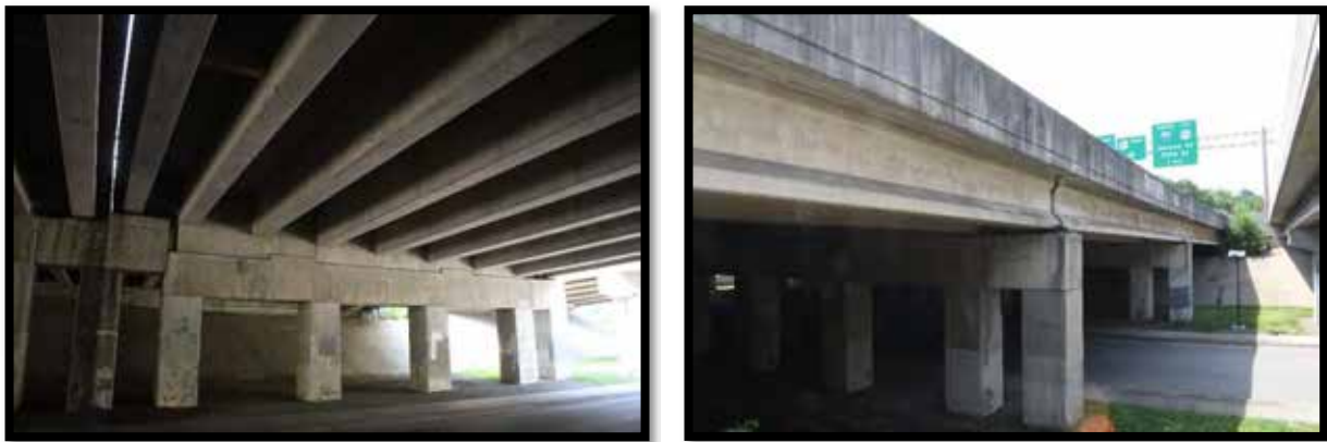
Plate 533. Bridge No. 059B00038R. Left: Bridge, looking at substructure. Right: Bridge, looking south. Note the additions of piers and girders on the outsides of the bridge.
