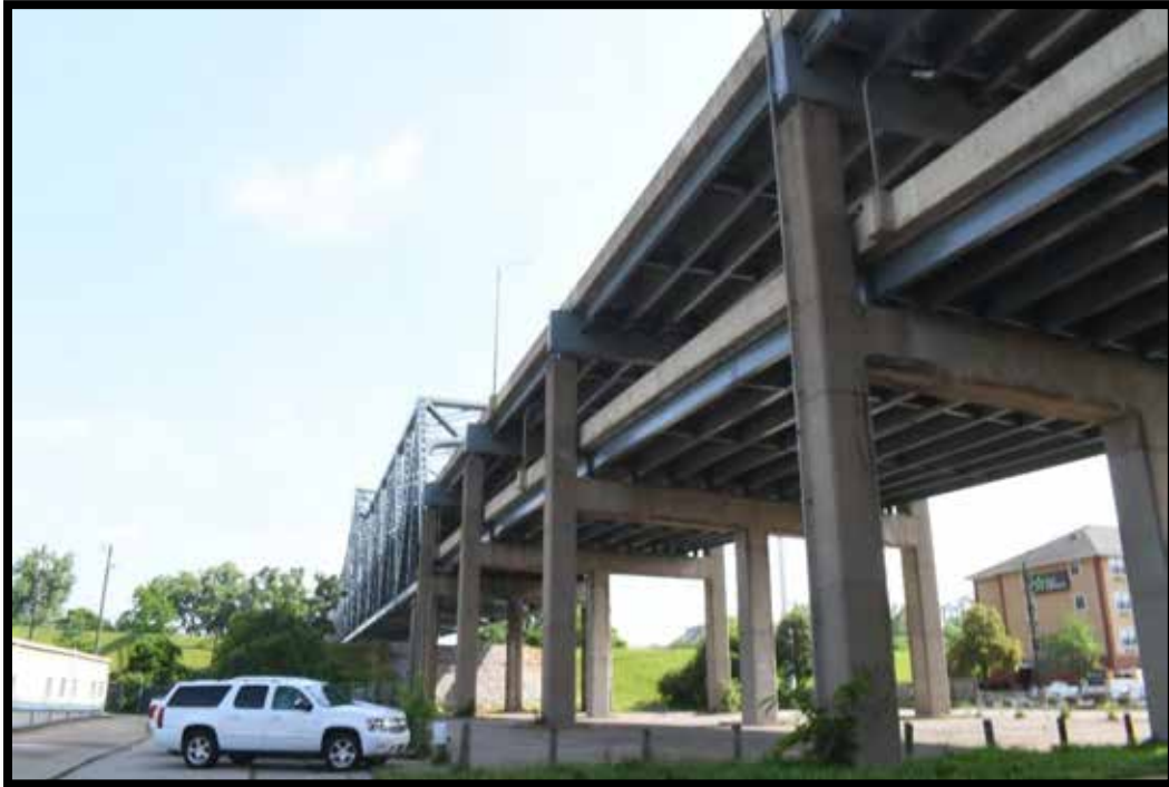
Plate 38. Brent Spence Bridge substructure, showing trusses and steel deck cantilevers, looking NE.
