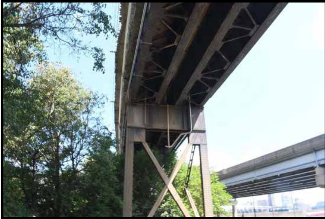
Plate 21. CSX Railroad Bridge No. 059R00633N (KEC-1062). Steel support truss and girders, looking north.
