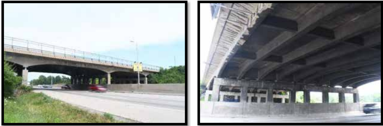
Plate 542. Bridge No 059B00047N. Left: Bridge, looking east. Right: Bridge, view of substructure.
