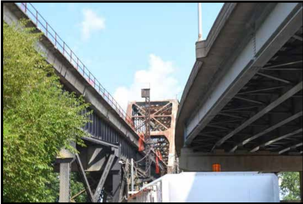
Plate 22. CSX Railroad Bridge No. 059R00633N (KEC-1062). Northern section of bridge, looking north.
