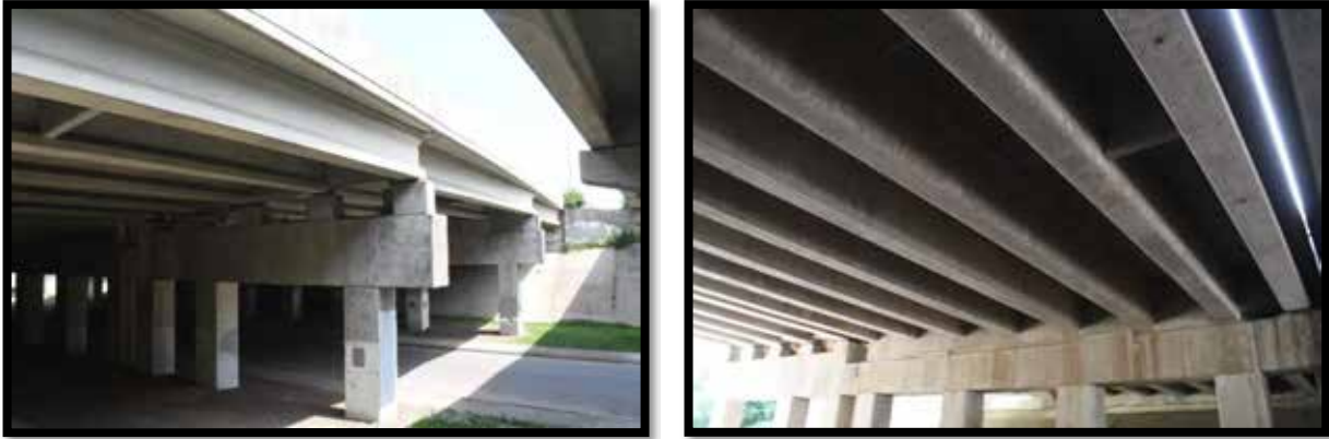
Plate 535. Bridge No. 059B00038L. Left: Bridge, looking north. Right: Bridge, looking at substructure. Note the additions of piers and girders on the outsides of the bridge.
