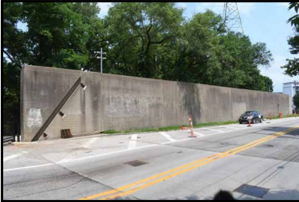
Plate 42. Covington Levee System within the APE. Southside of concrete levee wall north of Highway Avenue between Western Avenue and Wright Street, looking northeast.
