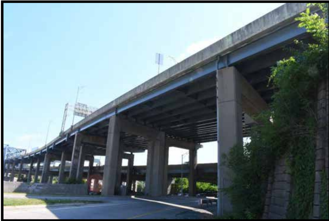
Plate 527. Bridge No. 059B00040N. Fifth Street section of Third, Fourth, and Fifth Street's overpass approach of I-75/71 to Brent Spence Bridge (Bridge No. 059B00046N), looking northeast.
