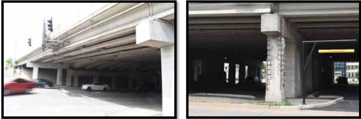
Plate 540. Bridge No. 059B00044L. Left: Bridge, view of substructure and arched girders on north section of bridge. Right: Representative view of deterioration, looking east.
