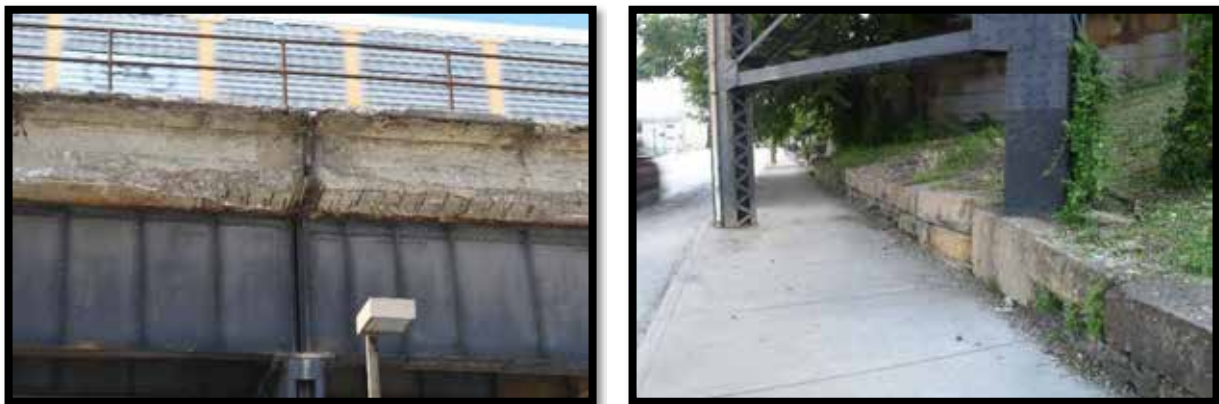
Plate 30. CSX Railroad Bridge No. 059R00610N (KEC-1065) (KEC-1065), Left: Representative example of bridge deterioration, looking SW. Right: Late nineteenth century stone wall adjacent to the south side of Fifth Street, below bridge support truss.
