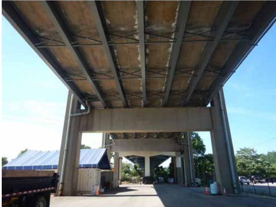
Photograph 9. View of the underside of the Brent Spence Bridge showing no signs of bat usage, looking south.
