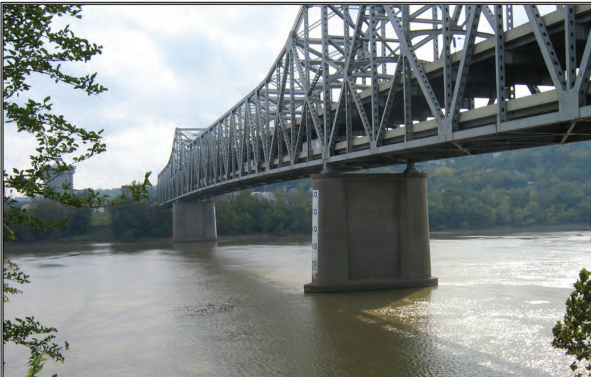
Photograph 2: Ohio River and existing Brent Spence Bridge (view from Ohio). Brent Spence Bridge Replacement and Rehabilitation Project. October 11, 2006.
