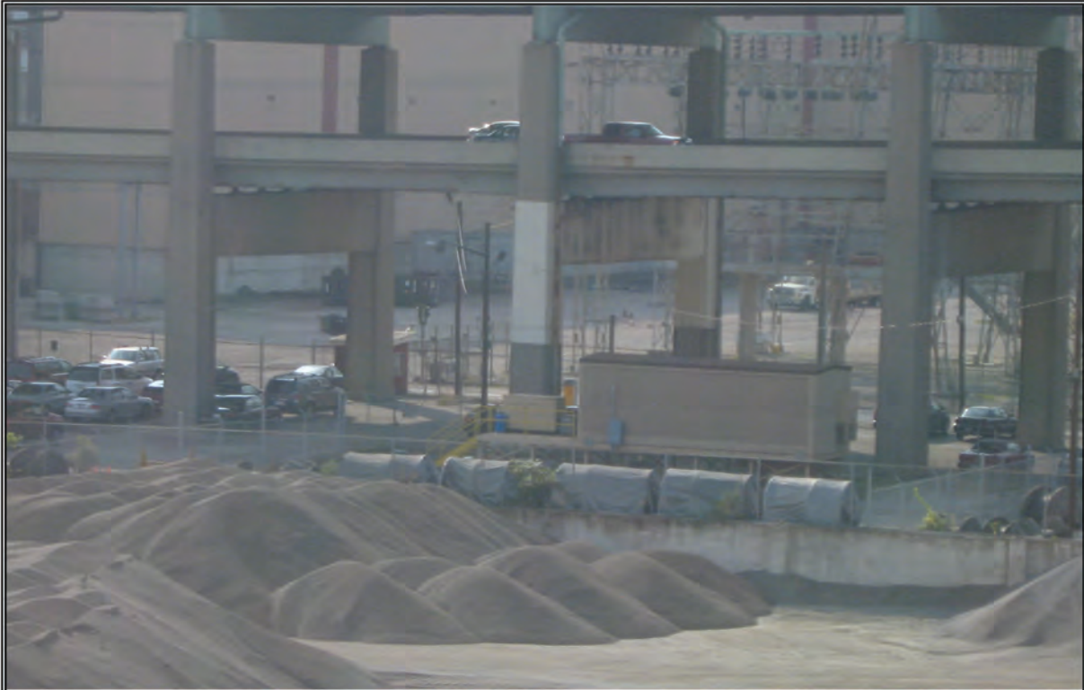
Photograph 7: Sand and gravel processing facility along Ohio River, adjacent to existing Brent Spence Bridge. Brent Spence Bridge Replacement and Rehabilitation Project. October 11, 2006.
