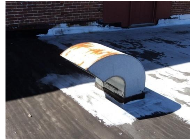
Photo 6: Elevator Ventilation Duct (noted Photo E-4 in Figure 4)
