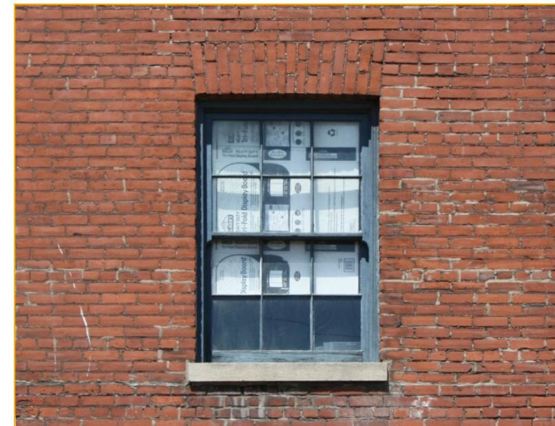
Photo 11: Minor Masonry Damage
