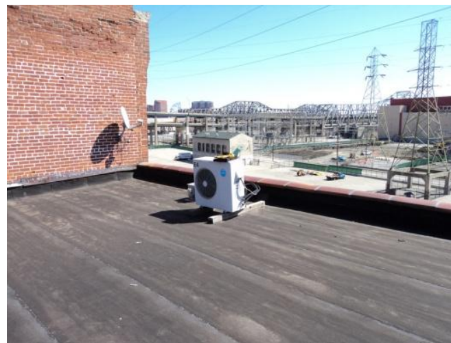
Photo 5: Computer Room Unit (noted Photo E-2 in Figure 4)
