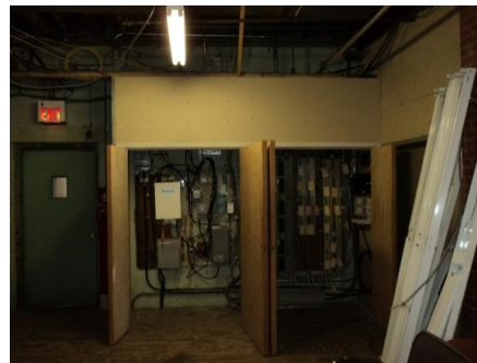
Photo 25: Main Communications Closet
