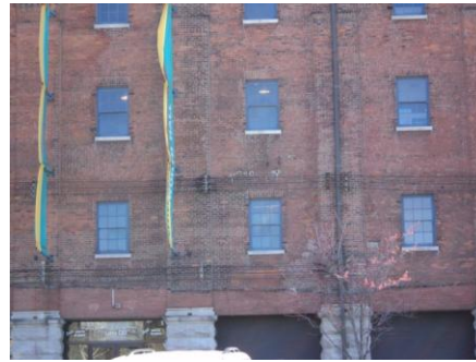
Photo 23: Elevator. Power Lines (top)
