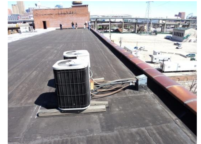
Photo 7: Condensing Units (noted Photo E-5 in Figure 4)
