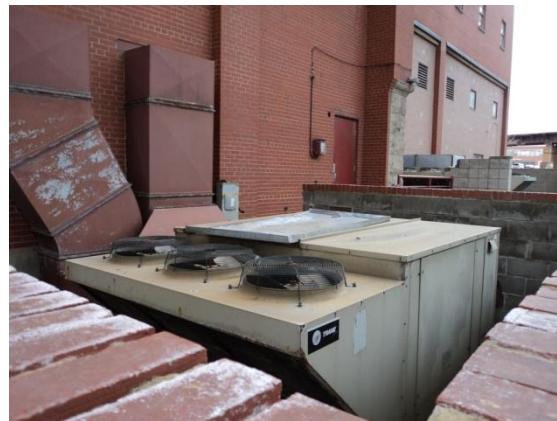
Photo 19: Grade mounted RTU
