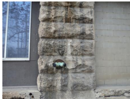
Photo 21: Fire Siamese Connection
