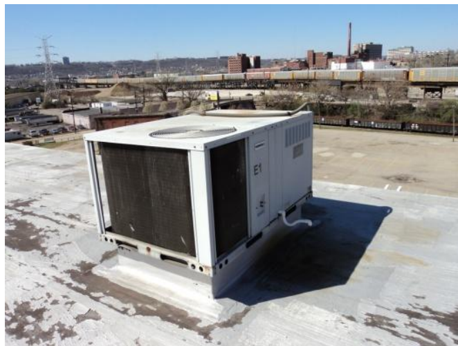
Photo 4: Packaged Rooftop Unit Condensing (noted Photo E-1 in Figure 4)
