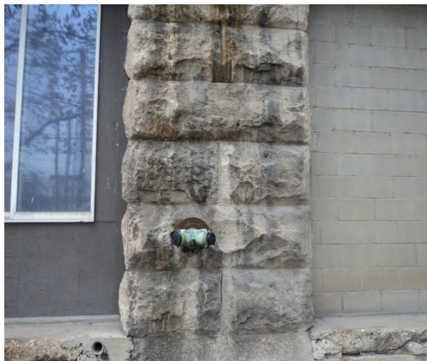
Photo 13: Fire Department Siamese connection
