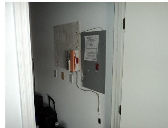
Photo 21: Area "B" 5 th floor breaker panel (noted Photo E-7 in Figure 19)
