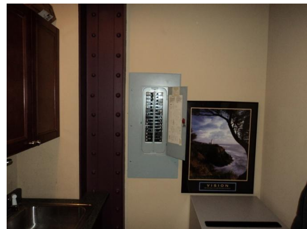
Photo 20: Area "B" 4 th floor breaker panel (noted Photo E-6 in Figure 18)
