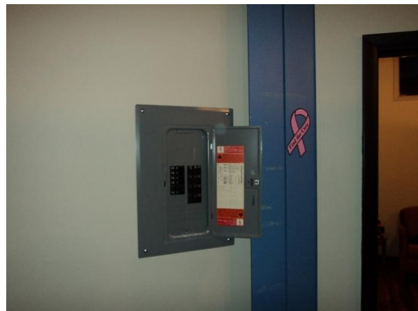
Photo 19: Area "B" 3 rd floor breaker panel (noted Photo E-5 in Figure 17)
