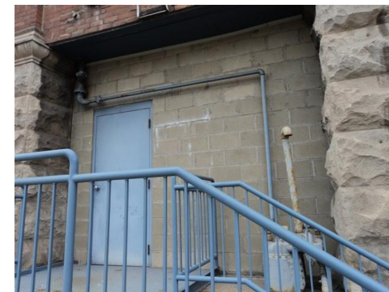
Photo 11: Area “F” incoming gas pipe
