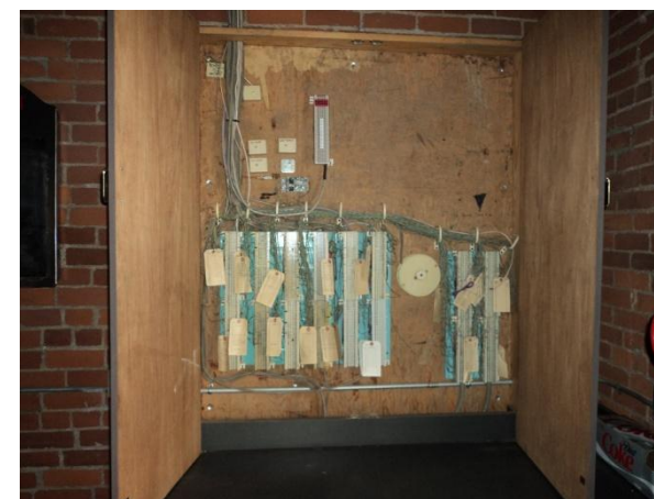
Photo 26: Main communications closet (noted Photo C-3 in Figure 15)
