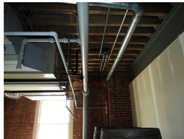
Photo 4: Typical indoor air-handling unit (noted Photo H-2 in Figure 16)
