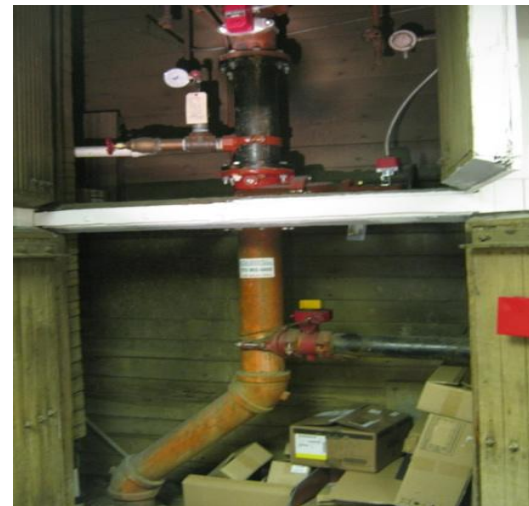
Photo 14: Area “B” valve closet (noted Photo FP-2 in Figure 14)
