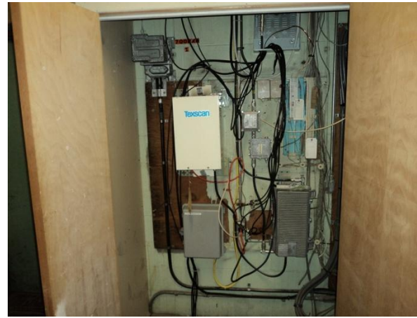
Photo 25: Main communications closet (noted Photo C-2 in Figure 15)
