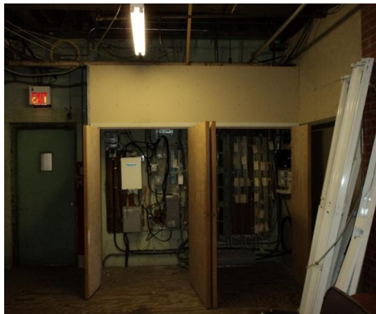
Photo 24: Main communications closet (noted Photo C-1 in Figure 15)
