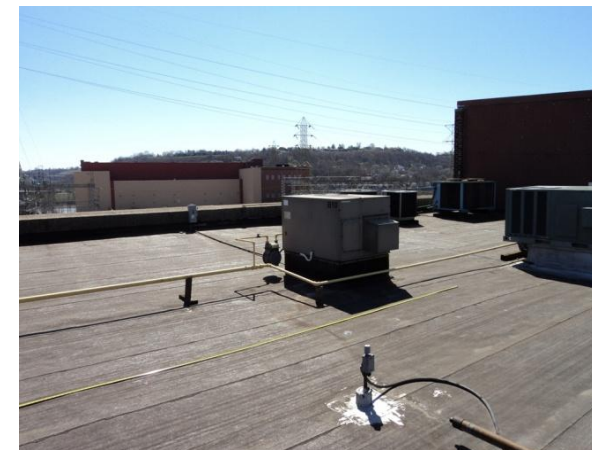
Photo 22: Area "B" power on roof
