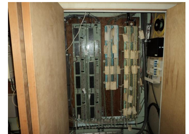
Photo 27: Sub-communications closet (noted Photo C-4 in Figure 17)
