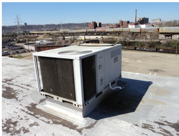
Photo 3: Typical rooftop unit
