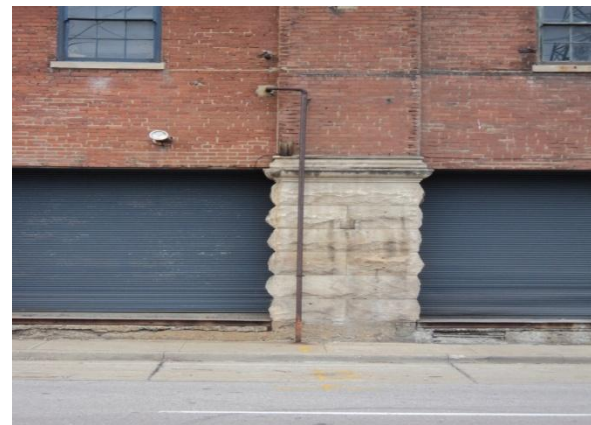
Photo 10: Area “D” incoming gas pipe
