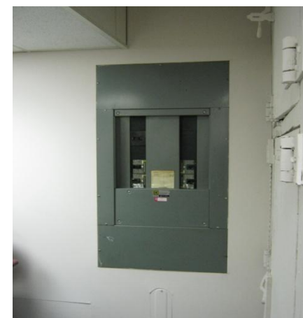
Photo 17: Area “B” main breaker panel (noted Photo E-3 in Figure 14)
