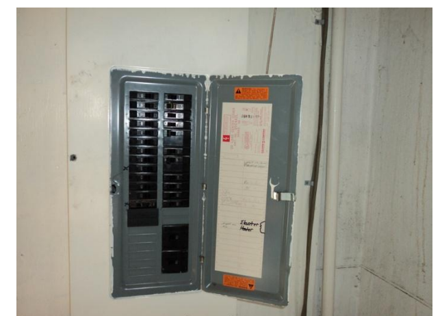
Photo 18: Area “B” 2 nd floor breaker panel (noted Photo E-4 in Figure 16)
