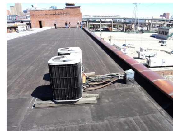
Photo 5: Typical air-cooled unit
