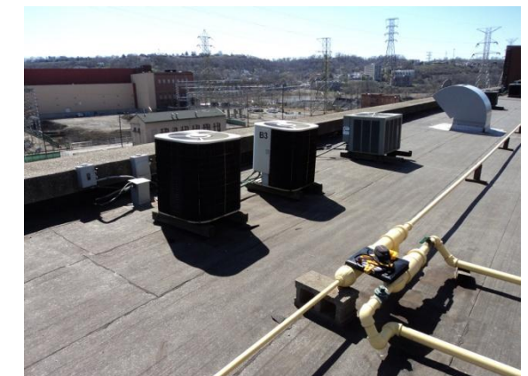
Photo 12: Area “B” gas piping on roof
