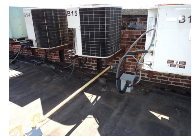
Photo 23: Area "B" power on roof
