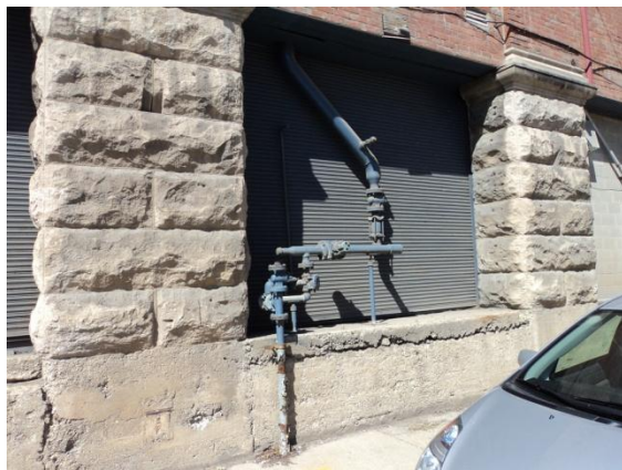
Photo 9: Area “B” incoming gas pipe (noted Photo G-1 in Figure 14)
