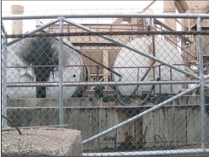
Site 65 - Valley Asphalt ASTs
