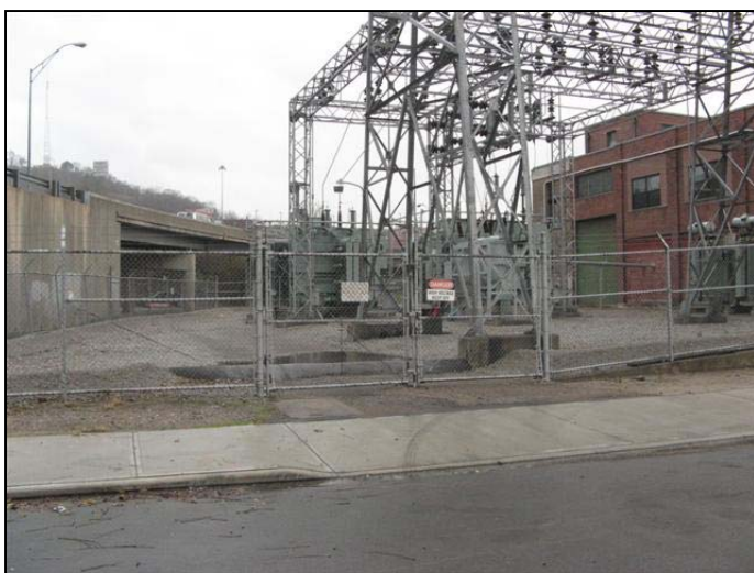
Site 2 - Duke Energy Substation. View from Buck Street
