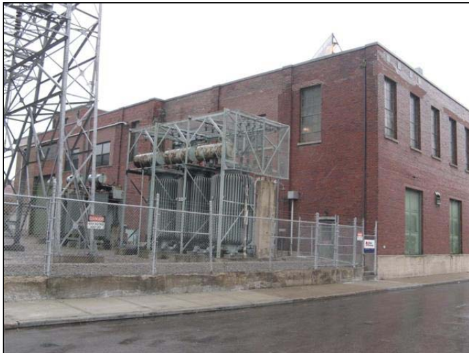
Site 2 - Duke Energy Substation
