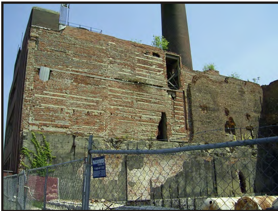
Plate B118. View of Hudepohl Brewery at 801 West 6th Street showing demolition, facing southeast.
