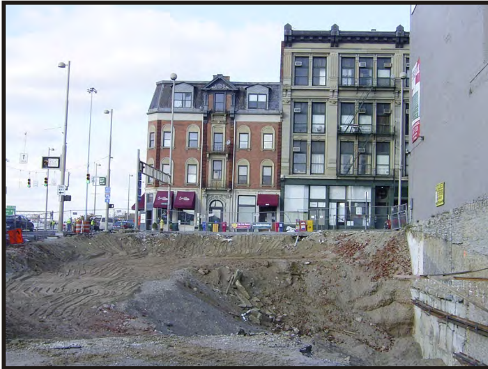
Plate B53. View of demolition site on West 4 th Street and Central Avenue within the West Fourth Street Historic District, facing north.
