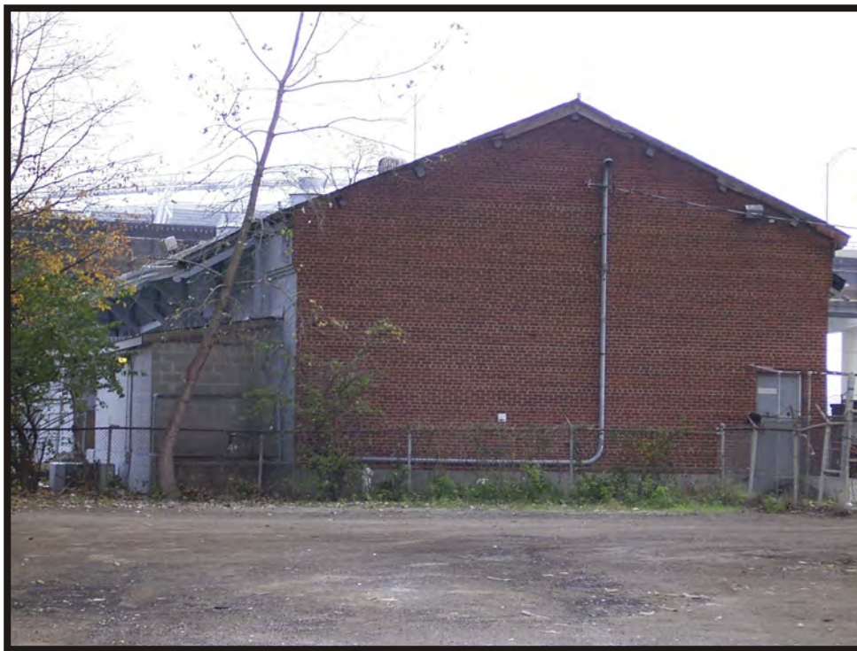
Plate B24. View of building at 603 West Pete Rose Way, facing east.
