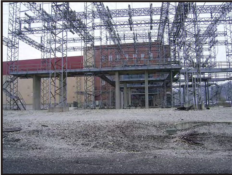
Plate B21. View of West End Electric Generating Station (HAM-5508-43), facing south.
