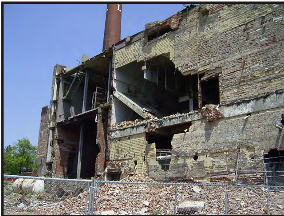
Plate B112. View of Hudepohl Brewery at 801 West 6th Street showing demolition, facing northeast.
