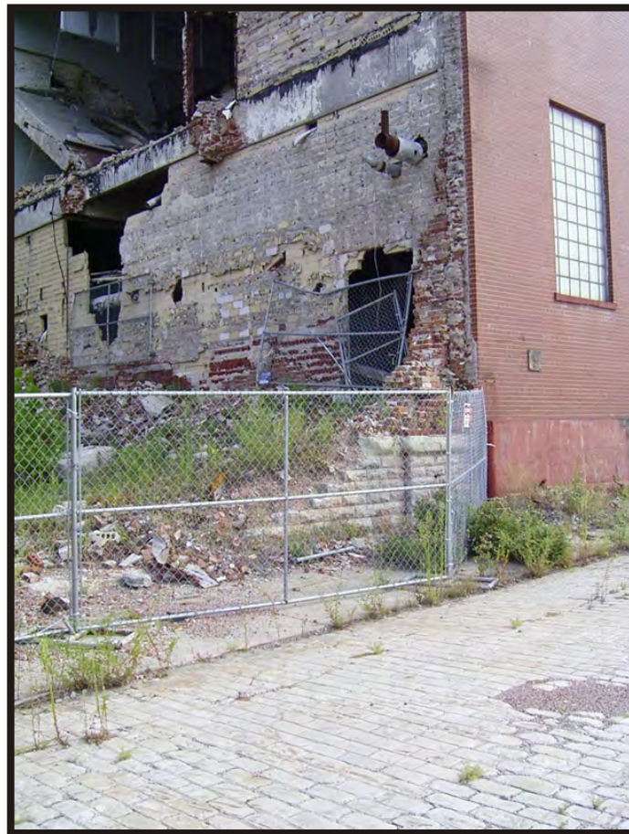
Plate B43. Detail of Hudepohl Brewing Company demolition site adjacent to 1960 addition, facing northeast.
