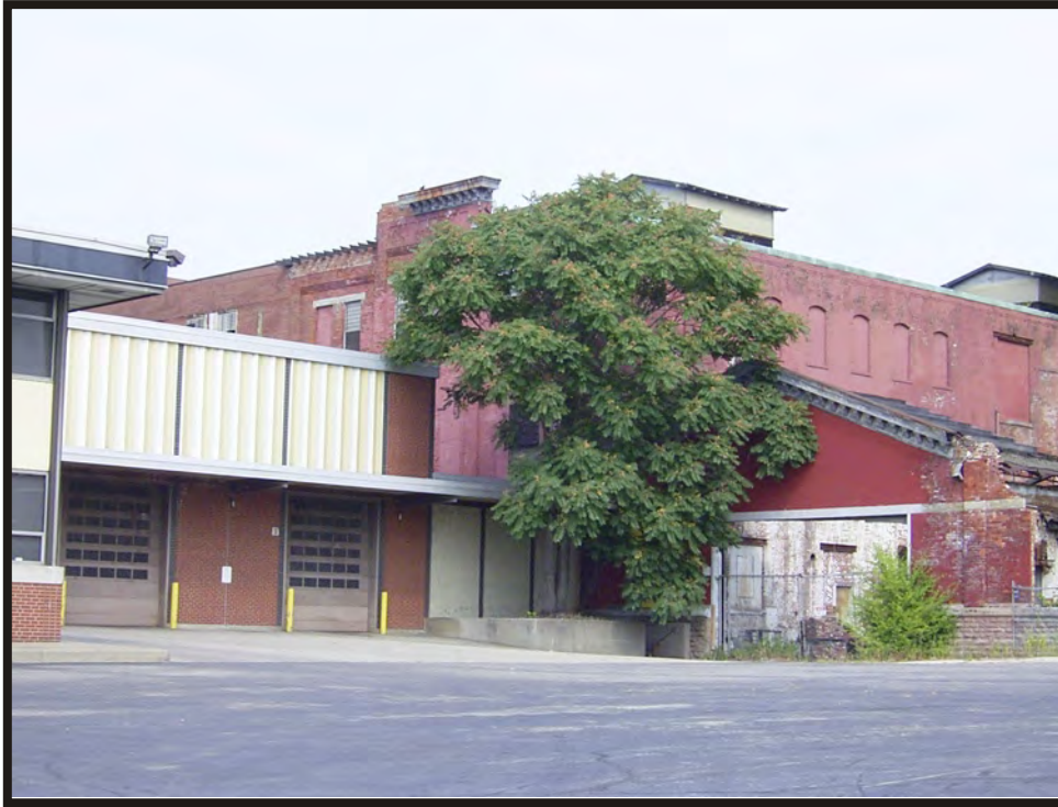
Plate B40. Detail of rear of Hudepohl Brewing Company complex, showing original Lackman Brewery buildings, facing northwest.
