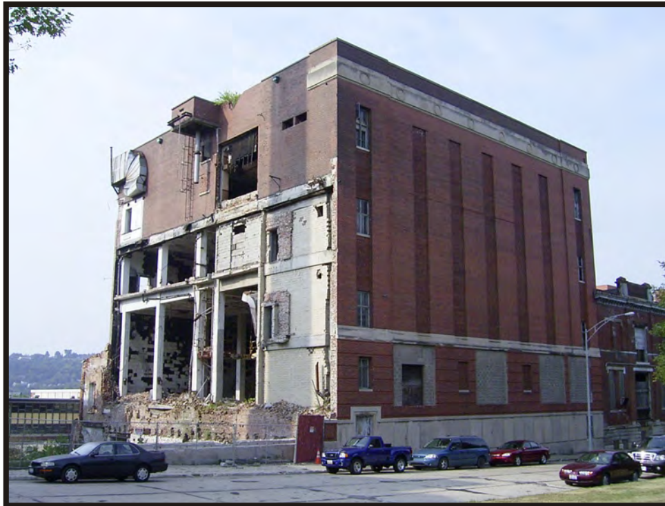
Plate B27. The Hudepohl Brewing Company 1947 addition and recent demolition, facing southwest.
