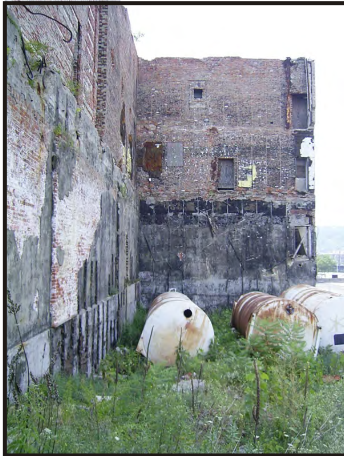
Plate B25. Detail of demolition site at the Hudepohl Brewing Company, facing south.
