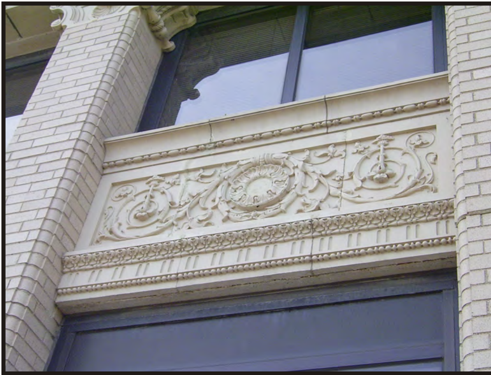
Plate B8. Detail of window frieze on northwest wing of Harriet Beecher Stowe School (HAM-1342-43), facing south.
