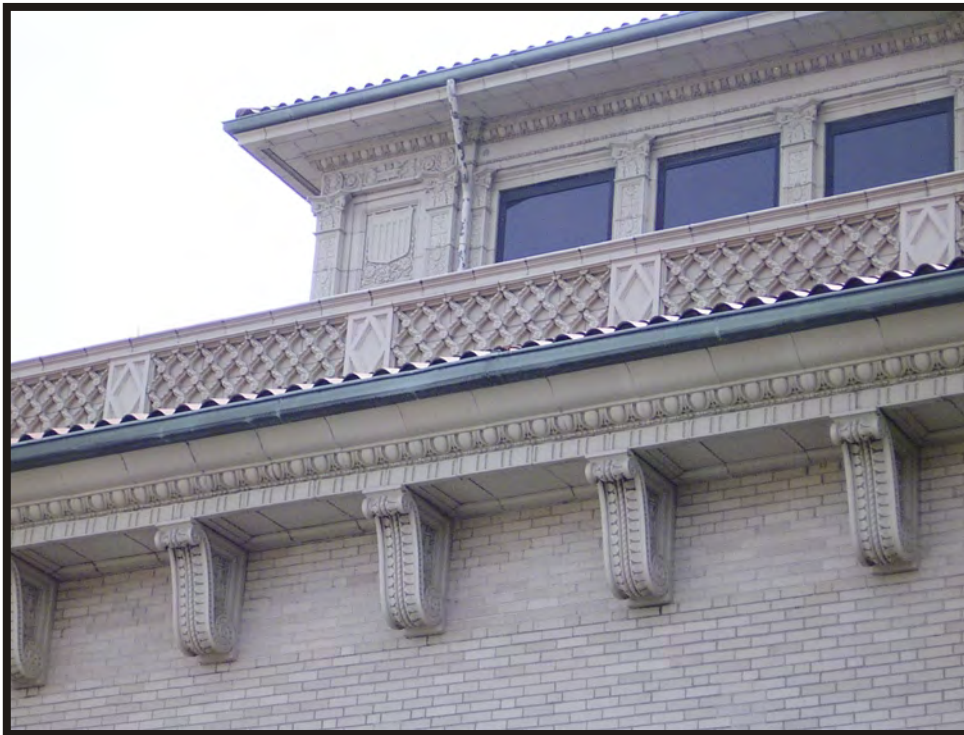
Plate B6. Detail of west façade of Harriet Beecher Stowe School (HAM-1342-43), facing east.
