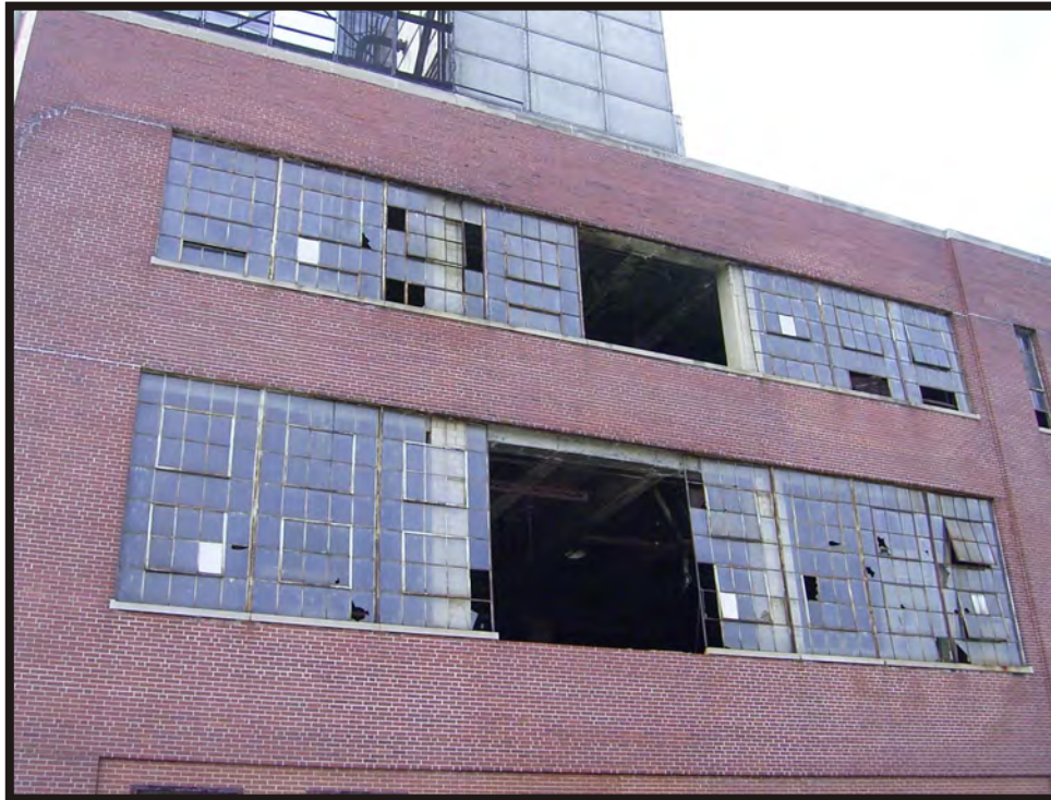
Plate B23. Detail of windows on the Hudepohl Brewing Company 1946 addition, facing south.
