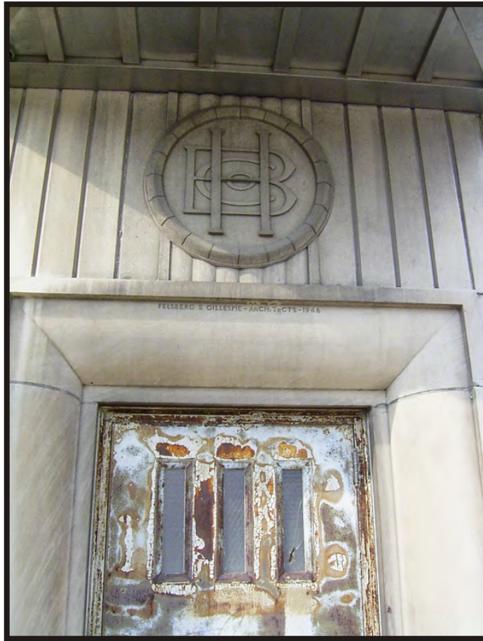
Plate B22. Detail of the Hudepohl Brewing Company logo, and the architect engraving on the main 1946 addition, facing southwest.
