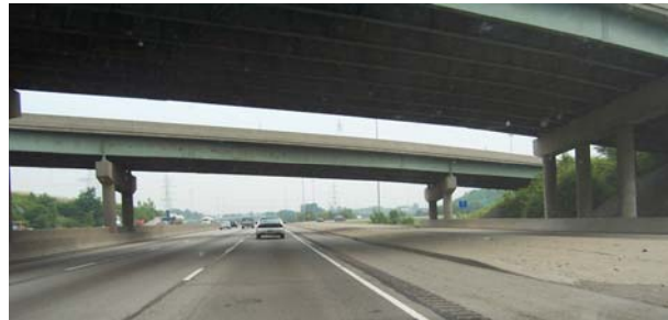
I-75 NB under SR126, showing proximity of bridge piers to I-75 existing edge of pavement.
