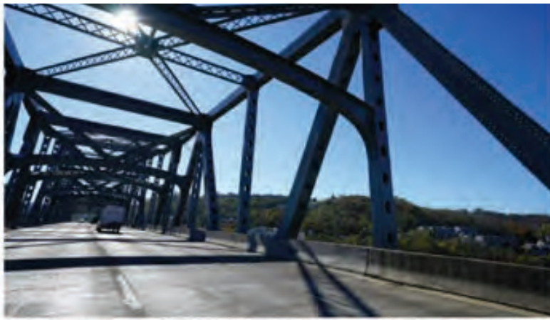
The Brent Spence Bridge - built in 1953 and maintained by the Kentucky Transportation Cabinet - transports about 160,000 vehicles a day over the Ohio River. That is twice the volume it was designed for. Kareem Elgazzar/The Enquirer
