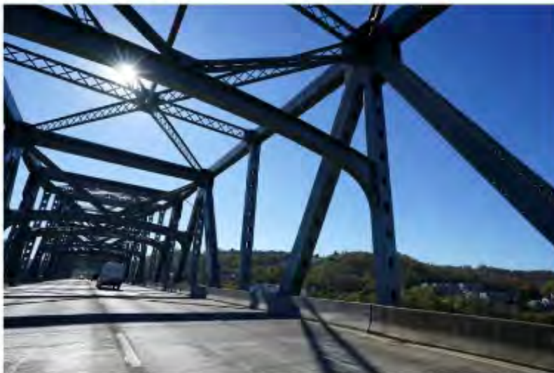
The Brent Spence Bridge - built in 1963 and maintained by the Kentucky Transportation Cabinet - transports about 160,000 vehicles a day over the Ohio River. That is twice the volume it was designed for. Kareem Elgazzar/The Enquirer
